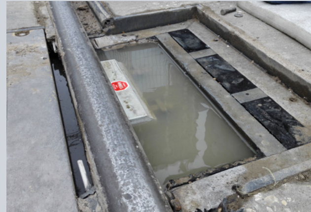
In Houston, wheel sensors must work reliably under water
