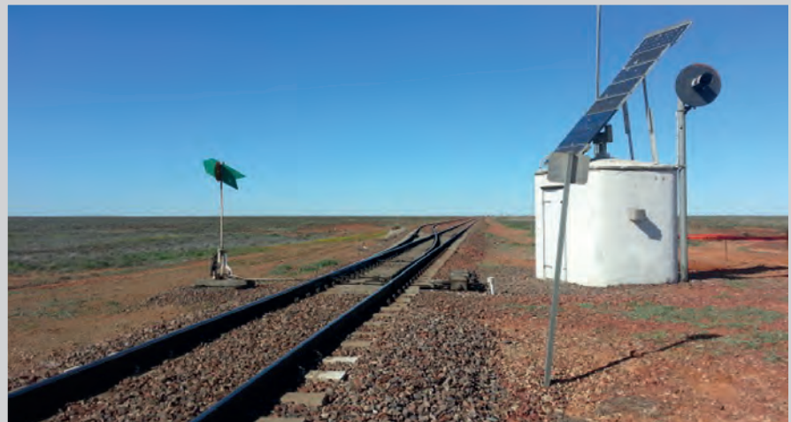
Figure 8: Modern signalling technology along the track in South Australia: ARTC aims for more efficiency by using open networks
