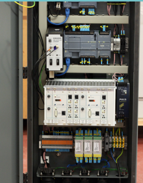
Cubical with ACS2000
